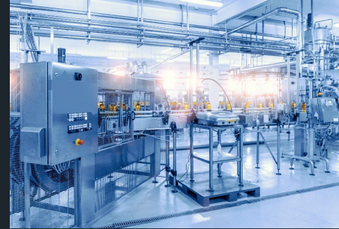
Industrial and Manufacturing
